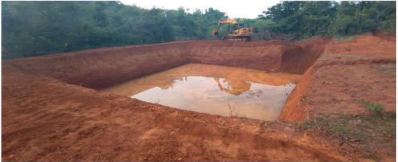
Creation of water pond at Honnavara Unit of Uttara Kannada District under RKVY RAFTAAR during 2020-21
